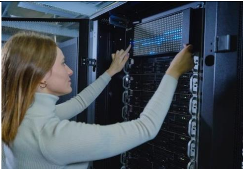
Caption: The Q.ANT NPU is available as a turnkey Native Processing Server (NPS), fully compatible and ready to plug into any HPC or data center. (image: Q.ANT GmbH)
